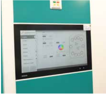
OT Control Panel
