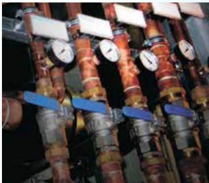
Medical Gas Pipeline Systems
