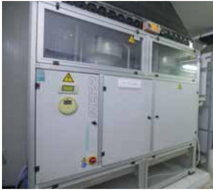
Hygiene Air Conditioning
